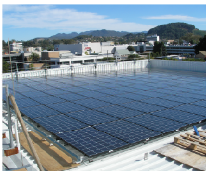
Photovoltaic installation, Rigby House, Coffs Harbour
